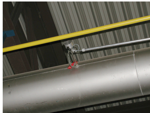
The nitrogen is also measured by SS 20.60 sensors.
