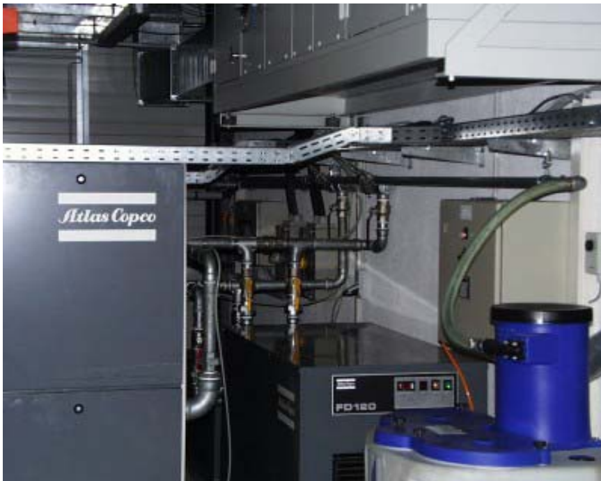
Compressor room of the company Glatt , a manufacturer of pharmaceutical machines. The SCHMIDT sensor SS 20.60 is mounted in a pipe at the ceiling (not visible).
