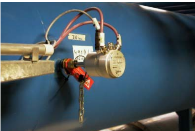
SCHMIDT SS 20.60 FB with Profibus Interface at the nitrogen intake pipe (diam. 700 mm) of a large ceramics kiln..
