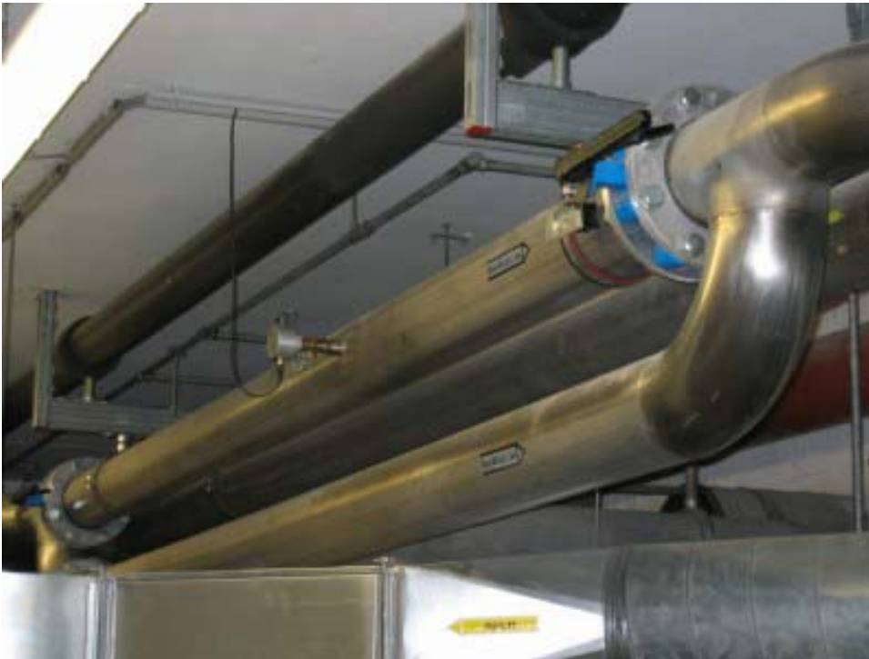
Measuring pipe with SS 20.60 at Swarovski AG (Austria) with a clever bypass solution.
