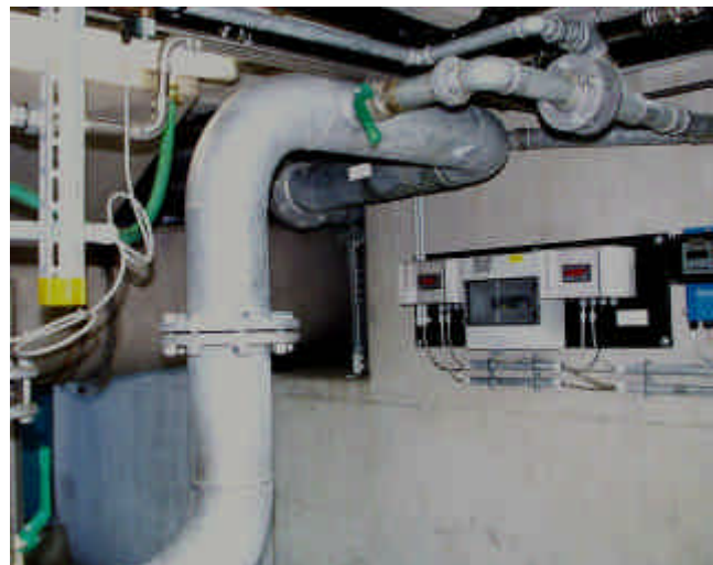
On-site display of volume flow
