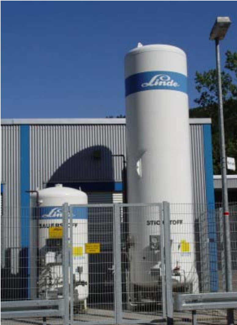
Nitrogen tank at a manufacturer of machine needles where 16 sensors SCHMIDT SS 20.60 are used for consumption measurement of nitrogen.
