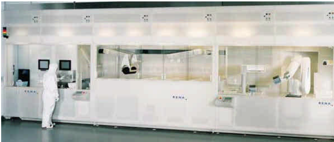
Wafer cleaning machine where the sensor SS 20.502 is used for control of volume-flow in a flow box. (not shown in picture)
