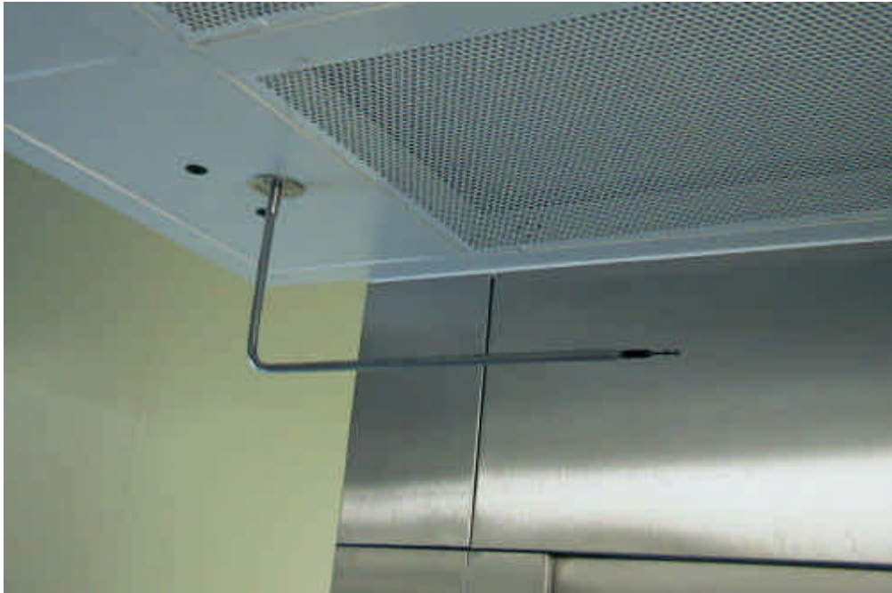
Laminar-flow Monitoring SS 20.502 under LF-Ceiling. The transformer is mounted in the false ceiling.
