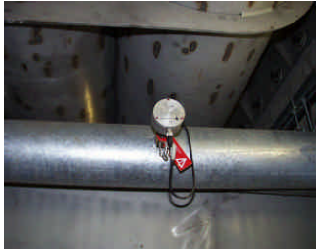
Sensor SS 20.60 in right main pipe
