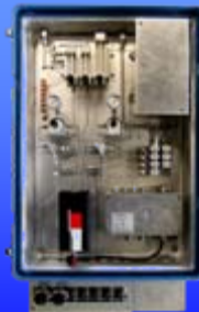
Simple Field Installation
