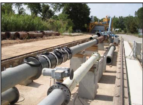
Assembly of several electromagnetic flowmeters for simultaneous calibration
