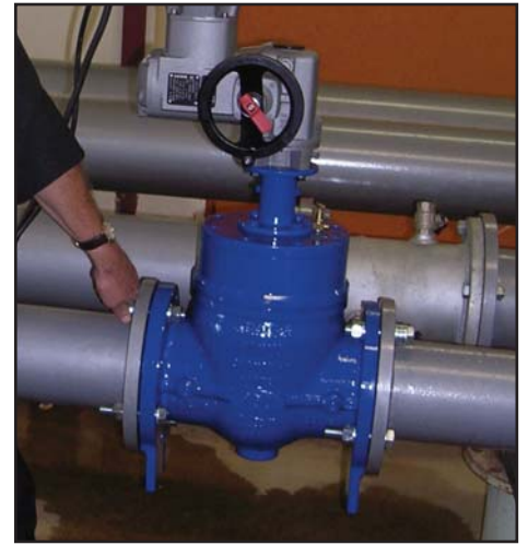
Hydraulic testing of a regulating valve ND150
