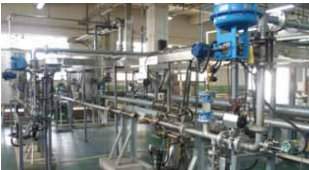
Calibration facility at Azbil Control Instruments (Dalian)
